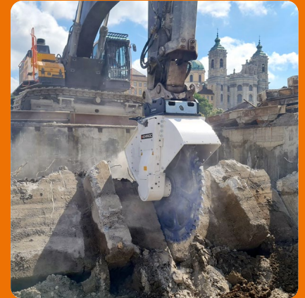
Massive concrete structures have to be demolished before a new multi-purpose quarter “Martinshöfe” can be built on a site below the basilica.
