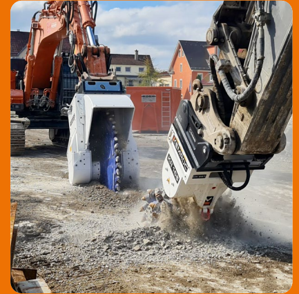
A 45 and a 60 tonne excavator with attachments from KEMROC play a major role at a CK Abbruch und Erdbau project in Weingarten.
