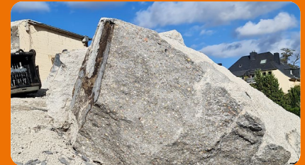
A comparatively unusual building material – completely unreinforced concrete. Using a hydraulic breaker, vibrations would have weakened the building.
