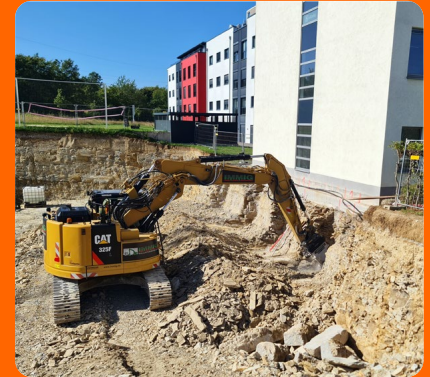
A 25-tonne crawler excavator and an EKT 100 drum cutter attachment from KEMROC during the excavation of a building in the Paderborn Technology Park.
