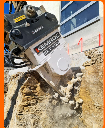
Without any vibrations to the building or its contents, rock below the façade is carefully and precisely milled out.
