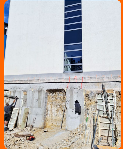
At set intervals, recesses are excavated, fitted with reinforcing formwork and then filled with concrete.
